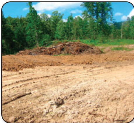
Over a mile of Mill Creek was bulldozed.
